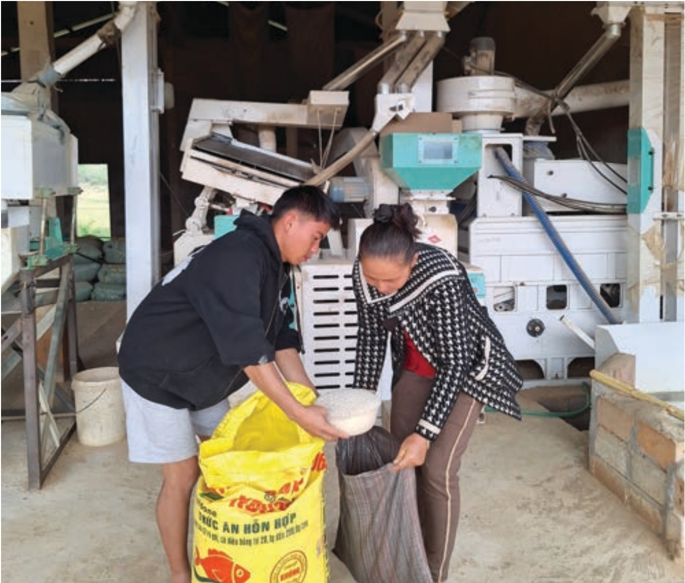
Rice milling, sorting and grading machine producing milled rice
